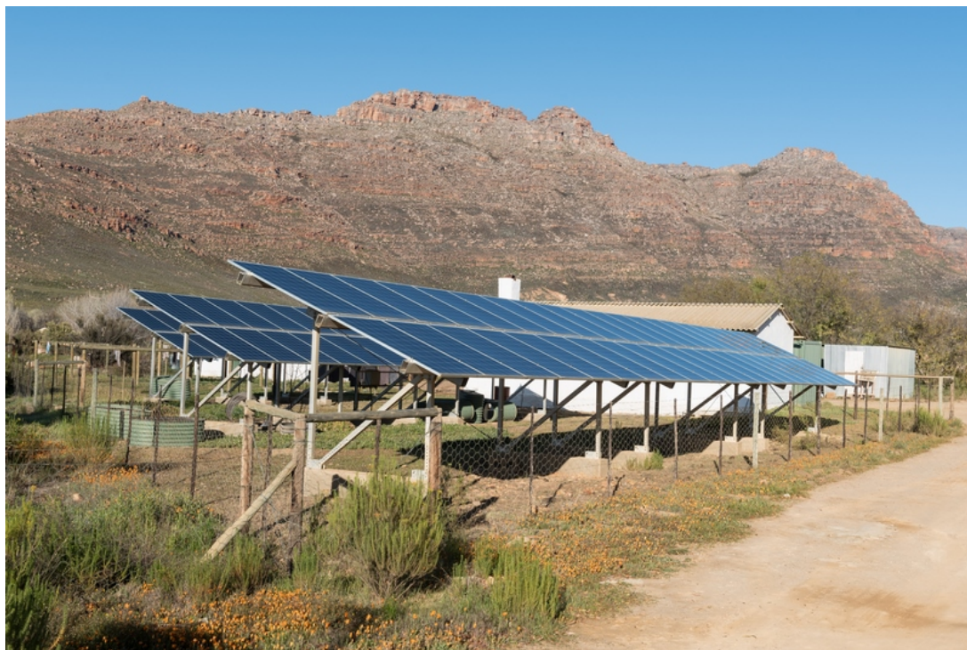
Kromrivier, South Africa – Sep 8, 2022: A solar power installation at Kromrivier Cederberg Park, a holiday resort in the Cederberg Mountains
